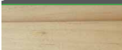
Pella's casement window after 7 months of exposure to moisture. 2
